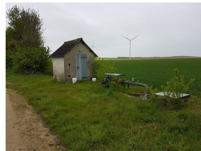
Photo 1. Station de pompage nord
