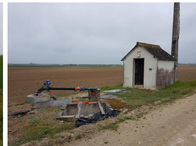
Photo 2. Station de pompage sud
